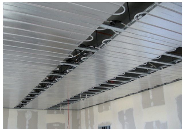
Fig. 75: Double function: Heating and cooling in the ceiling area
