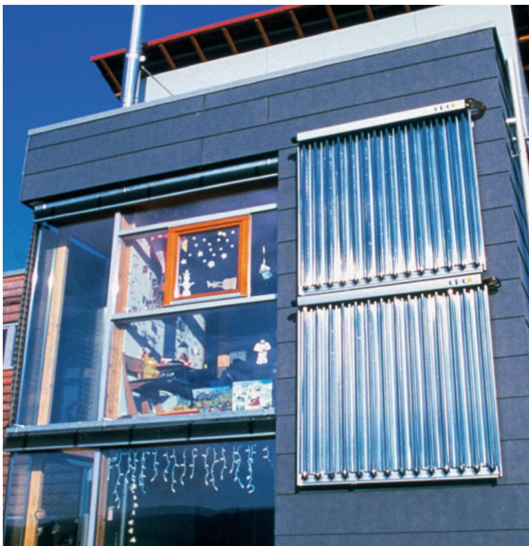
Fig. 53: Example of vacuum tube collector installations
