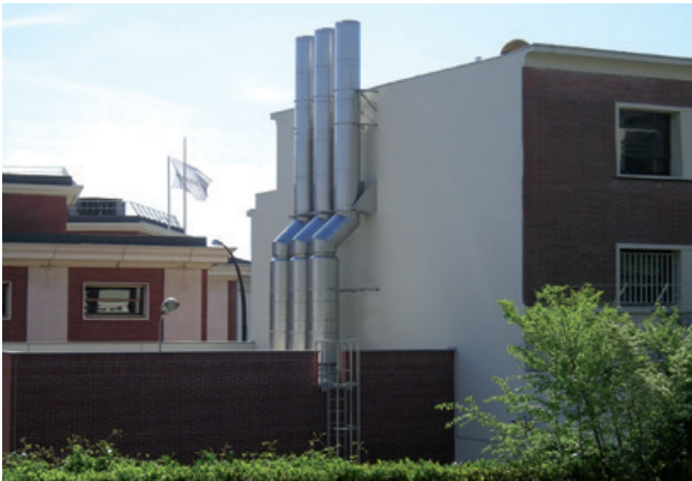
Fig. 94: Stainless steel flue gas systems in firing systems operated by combustion engine
