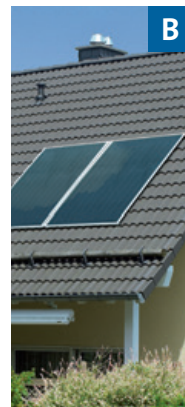
Solar thermal system for domestic hot water
