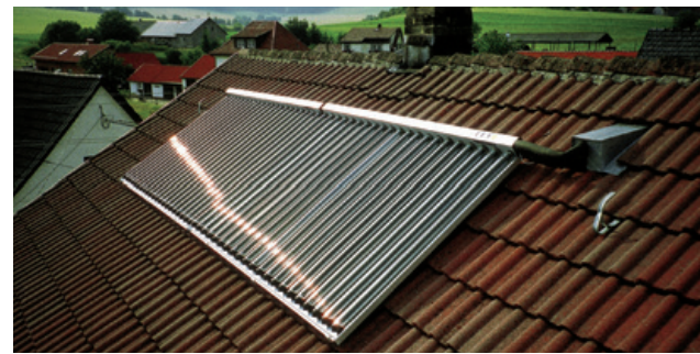
Fig. 52: Example of solar installations – Vacuum tube collector
