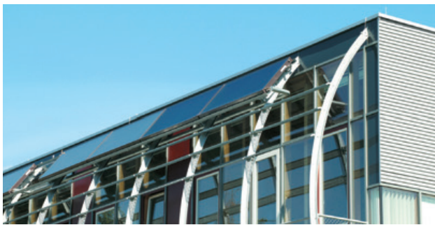
Fig. 51: Example of solar installations – Flat plate collector
