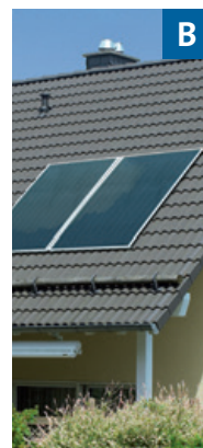
Solar thermal system for domestic hot water
